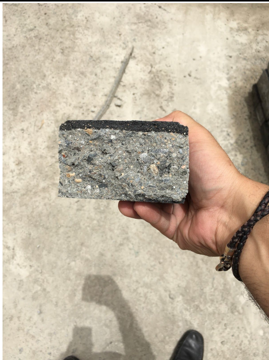
Densely packed concrete with 10mm and below aggregates. Substantial top layer for wearing surface.
